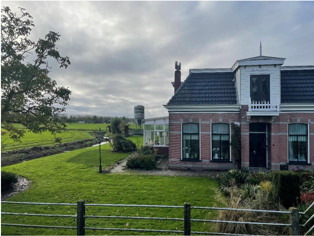
Figure 108. Near Eibersburen view on old Farmhouse with clear visible damage which has a geodetic marker
